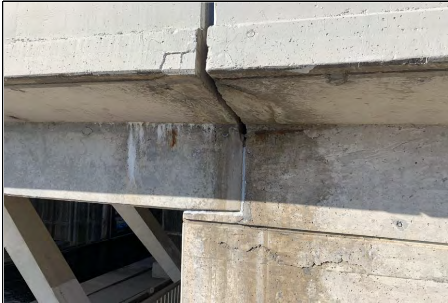
Photo 5: Rebar Exposure and Leaking at NE Expansion Joint
