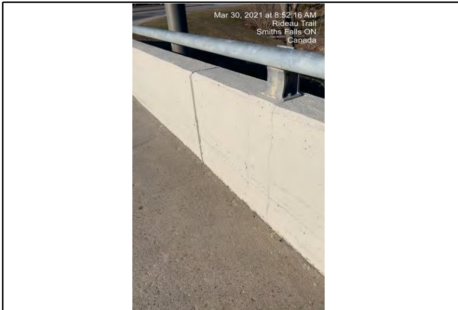
Photo 7: Cracks in Interior Parapet
