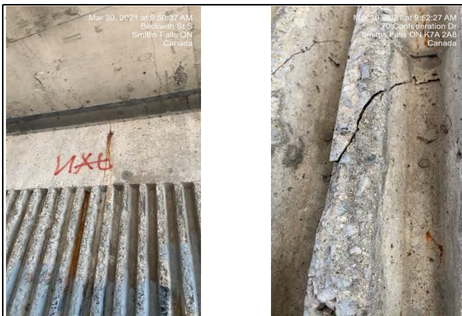
Photo 8: Spall and Crack at North Abutment Wall
