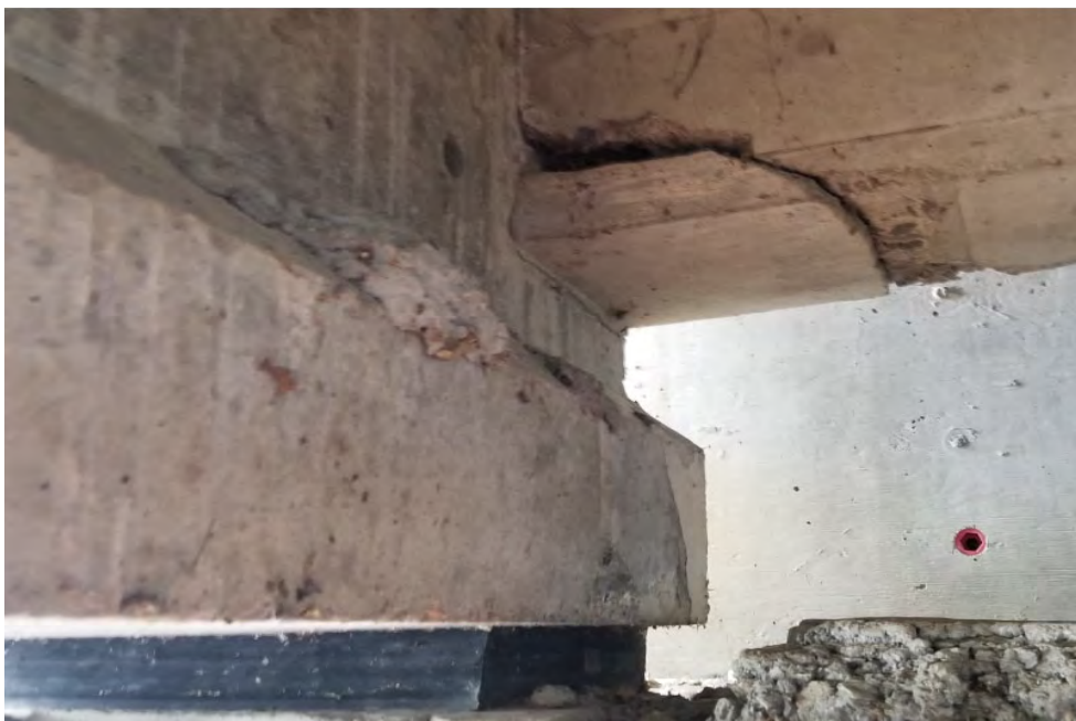
Photo 16: Concrete Spalling and Severe Cracking at Girder Bridging
