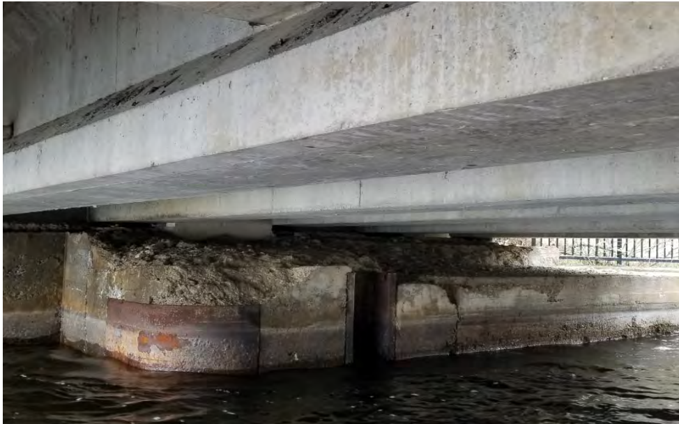
Photo 15: Delamination and Cracks at North Abutment
