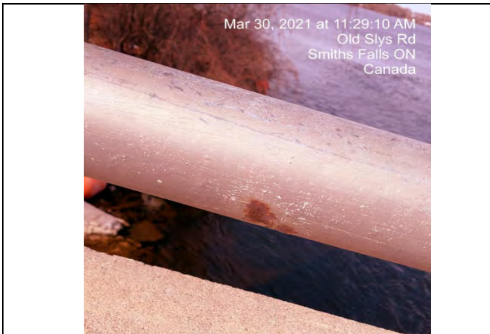
Photo 10: Rust on Railing
