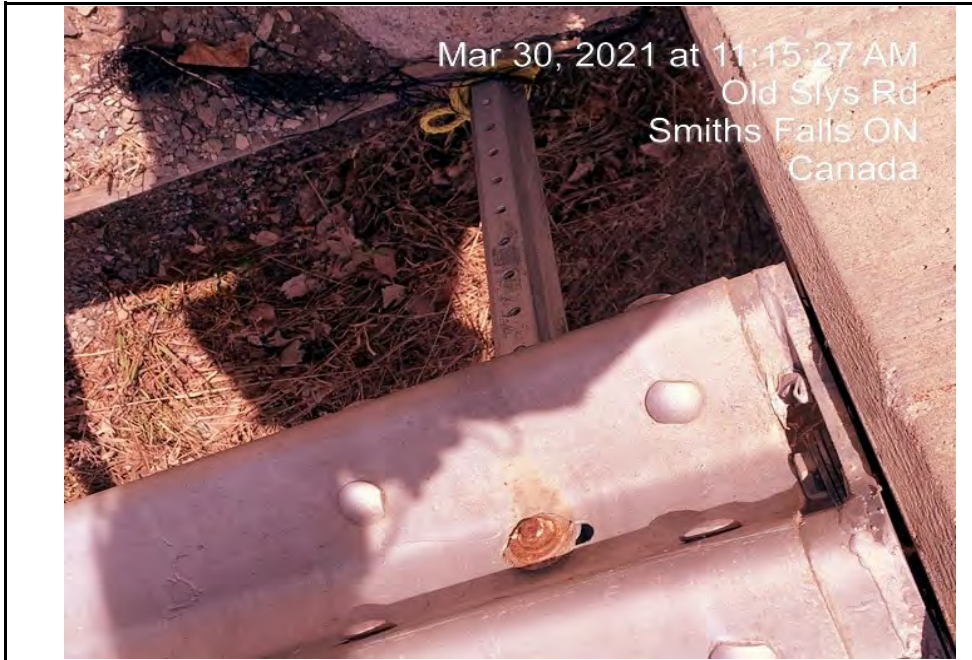
Photo 9: Rusted Bolt at N/W Guardrail
