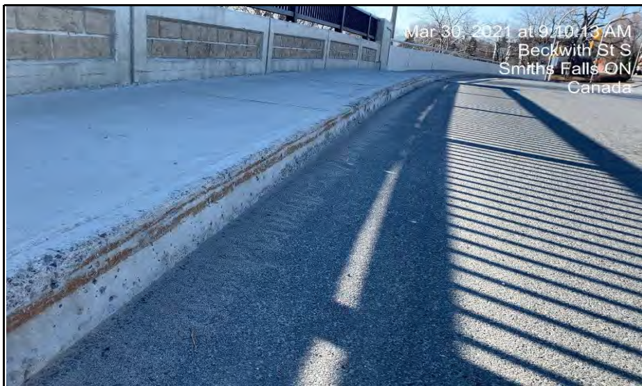
Photo 4: Concrete Sidewalk Delamination
