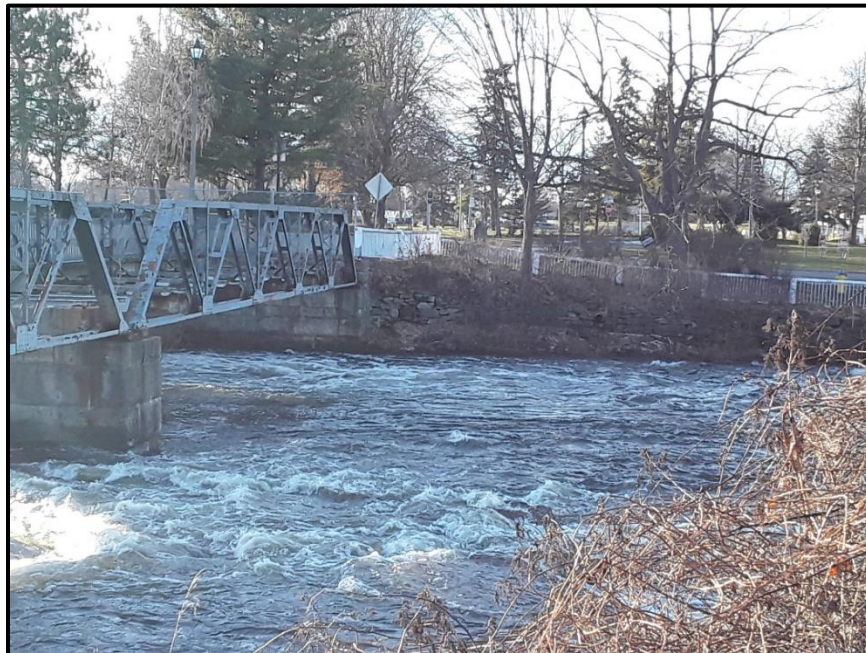
Image 10. View of the western footing of the Confederation Drive bridge as seen from the east bank of the waste water channel, facing west. (PR21-059D070)
