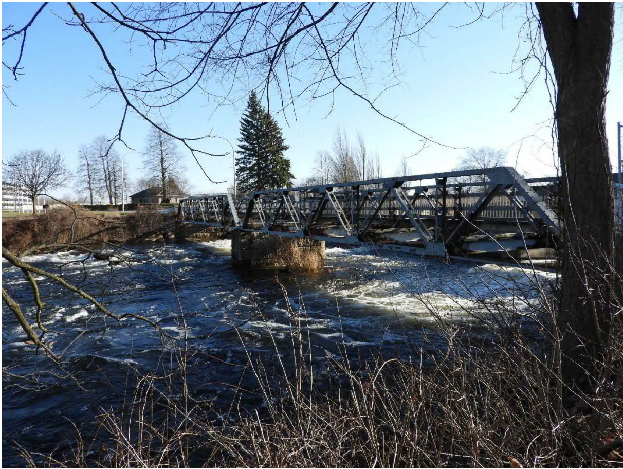
Photo 3: Full view of the entire Confederation Drive bridge from the northwestern bank. Below the bridge flows a portion of the Rideau River, diverted to the north from the implementation of a federal dam.
