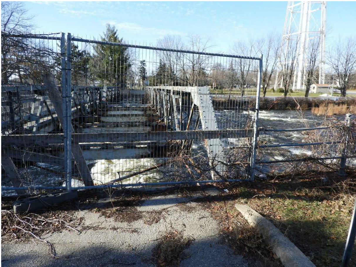
Photo 2: Barricaded eastern entrance to the Confederation Drive bridge, implemented in 2015 due to unsafe structural conditions; however, this barricade also limited access and obstructed view to some portions of the bridge during the 2021 field investigations.
