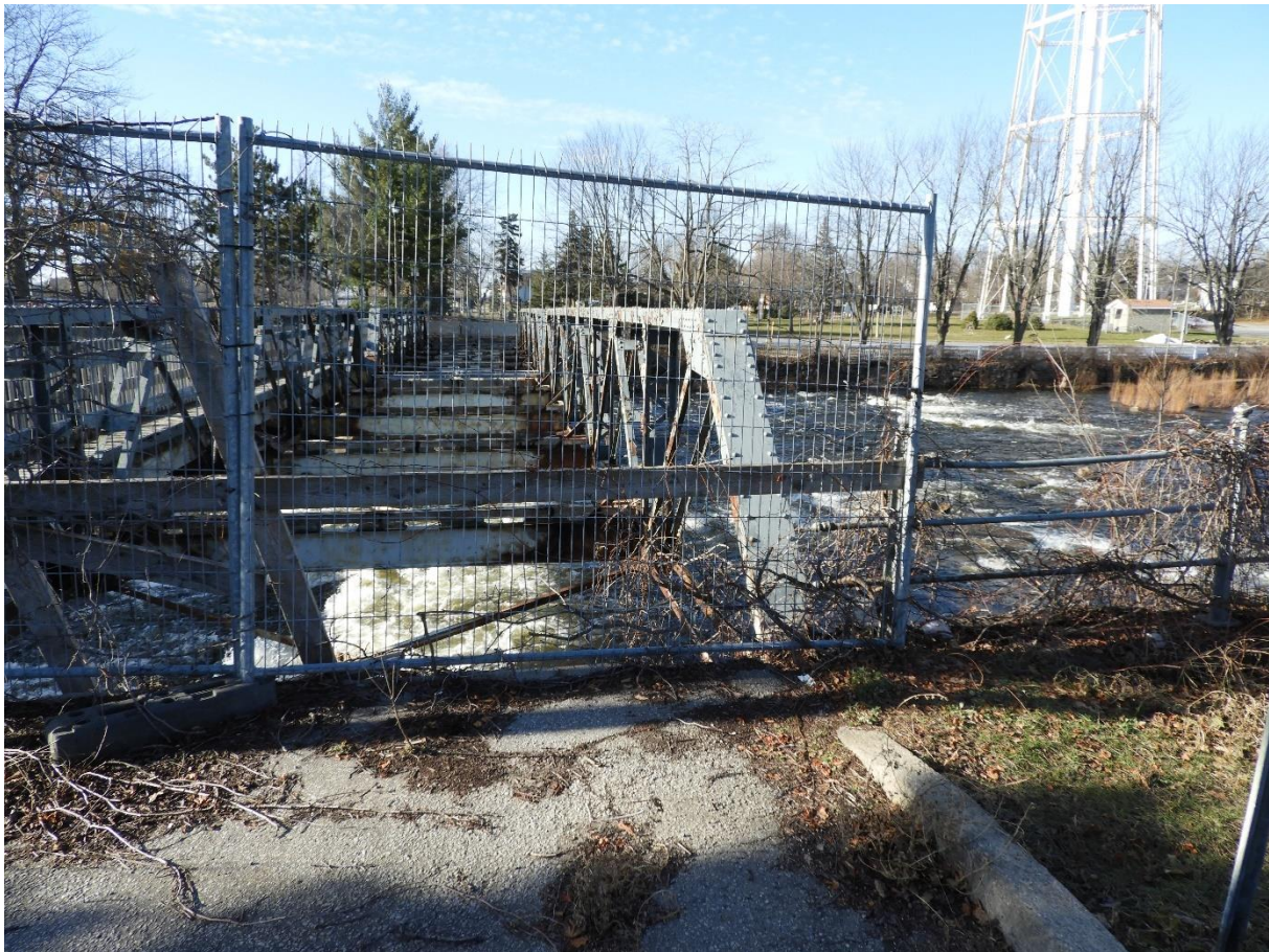
Photo 2: Barricaded eastern entrance to the Confederation Drive bridge, implemented in 2015 due to unsafe structural conditions; however, this barricade also limited access and obstructed view to some portions of the bridge during the 2021 field investigations.
