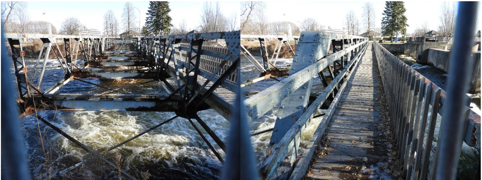
Photo 6: Sections of the Confederation Drive bridge structure where existing timber deck was removed from the bridge (left) and the remnants of the wooden pedestrian pathway (right).
