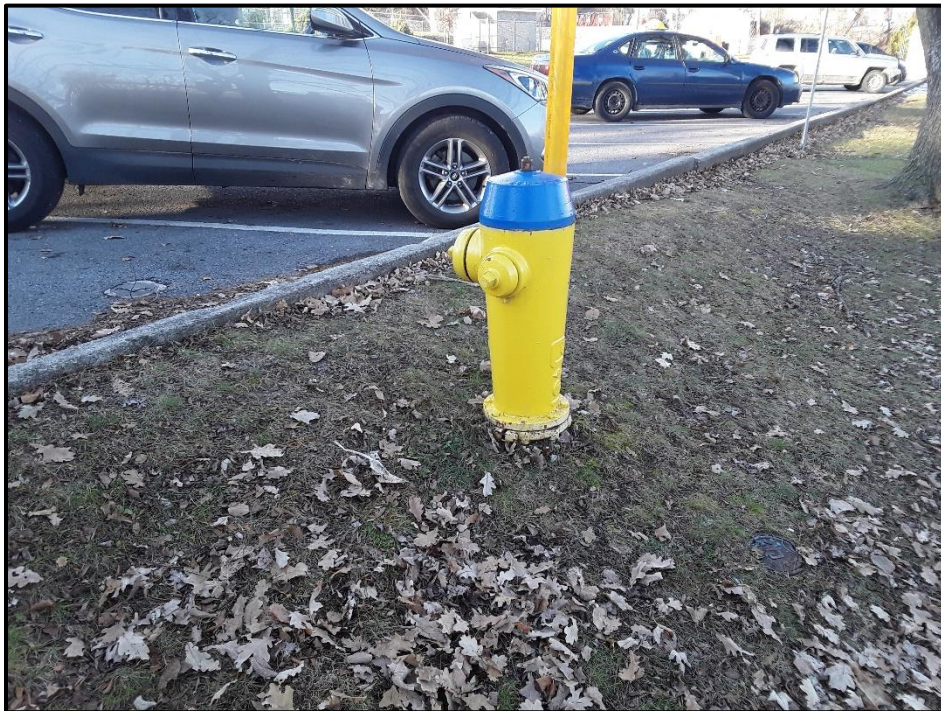
Image 6. View of a fire hydrant and water main valves in the northwest part of the study area, facing north. (PR21-059D030)
