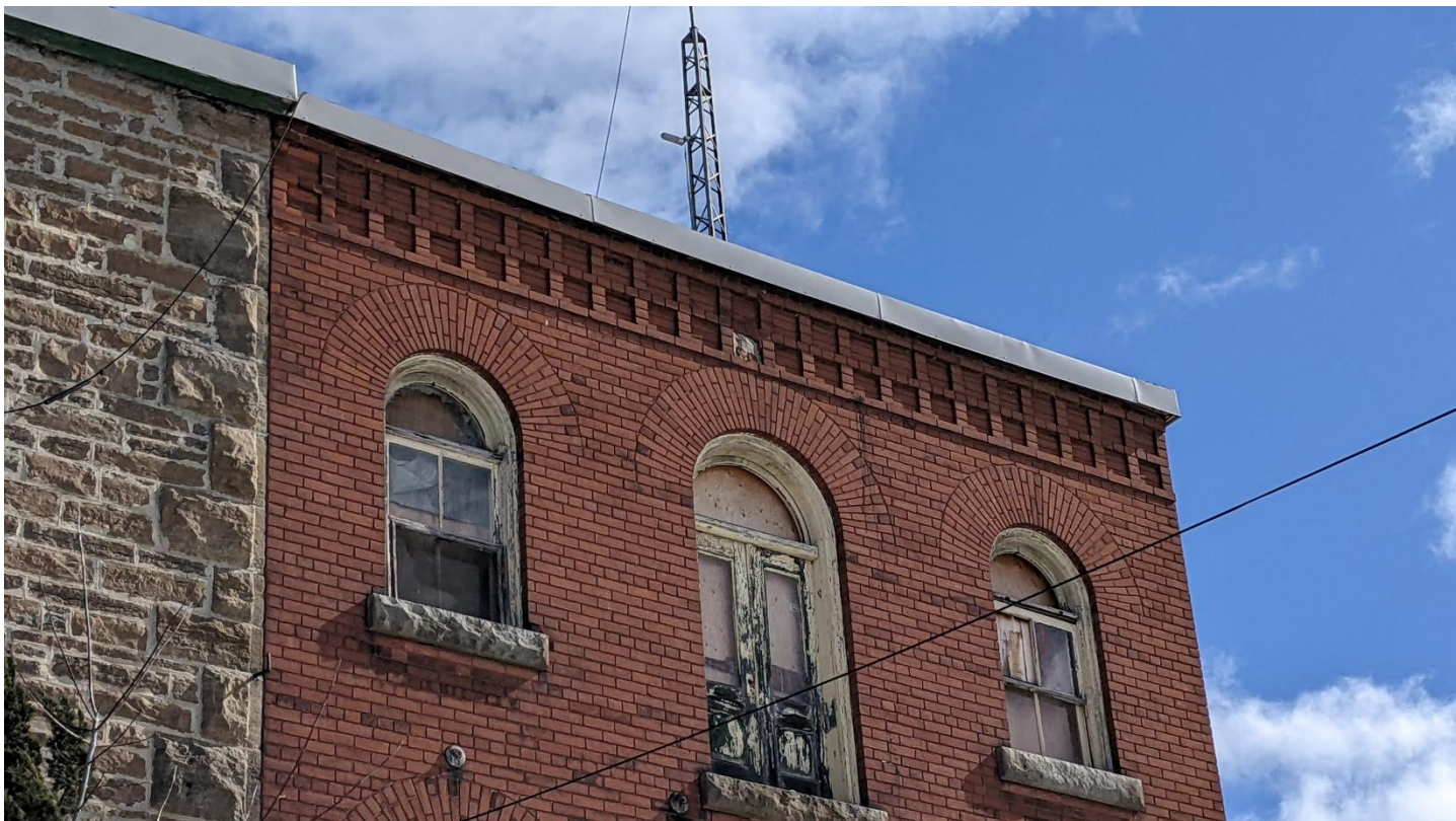
4 Detailed view of Building 2's intricate brickwork, including radiating voussoirs above the arched windows. The decorative brick cornice visible at the building's roofline. Image: MTBA.
