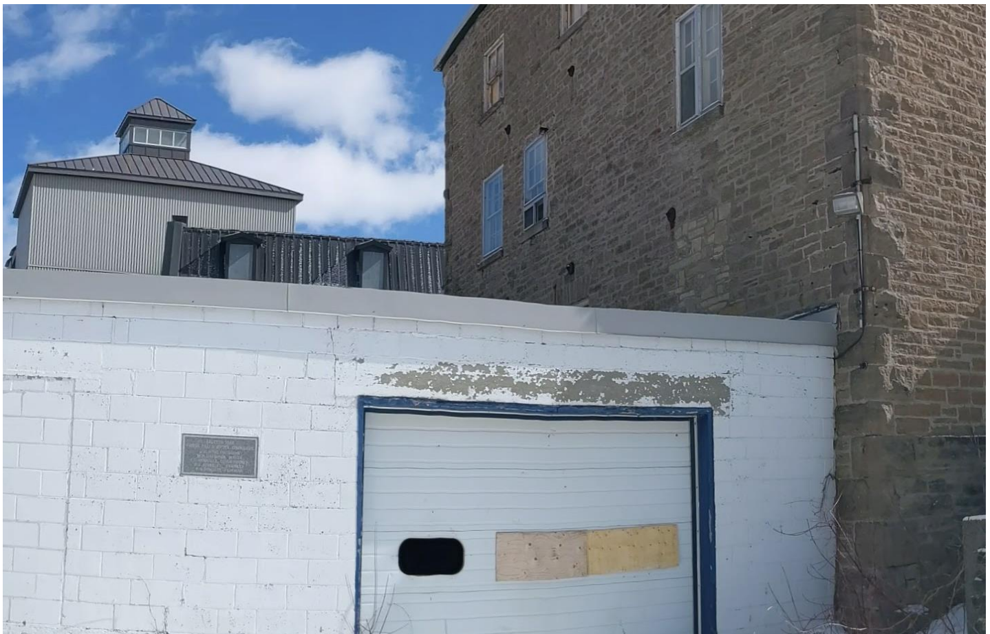
7 Building 4 (left), located just north of Building 1, built in 1954. The building's concrete block construction and garage openings illustrate its function and use. The building's inscription plaque is a character-defining element. Image: MTBA.
