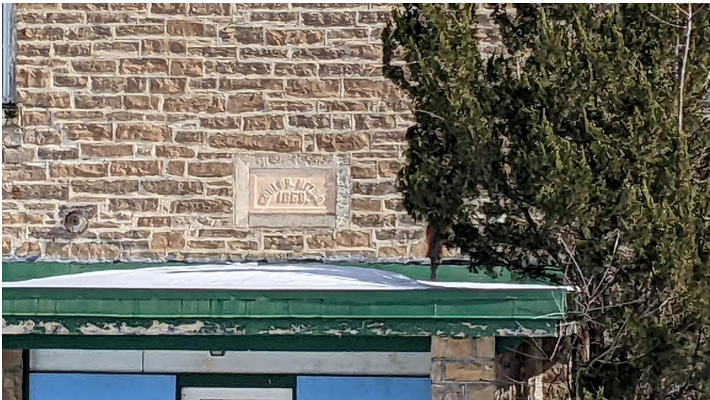
2 Date stone, bearing inscription 1868 on Building 1, above the west entrance extrusion with masonry piers. Image: MTBA.
