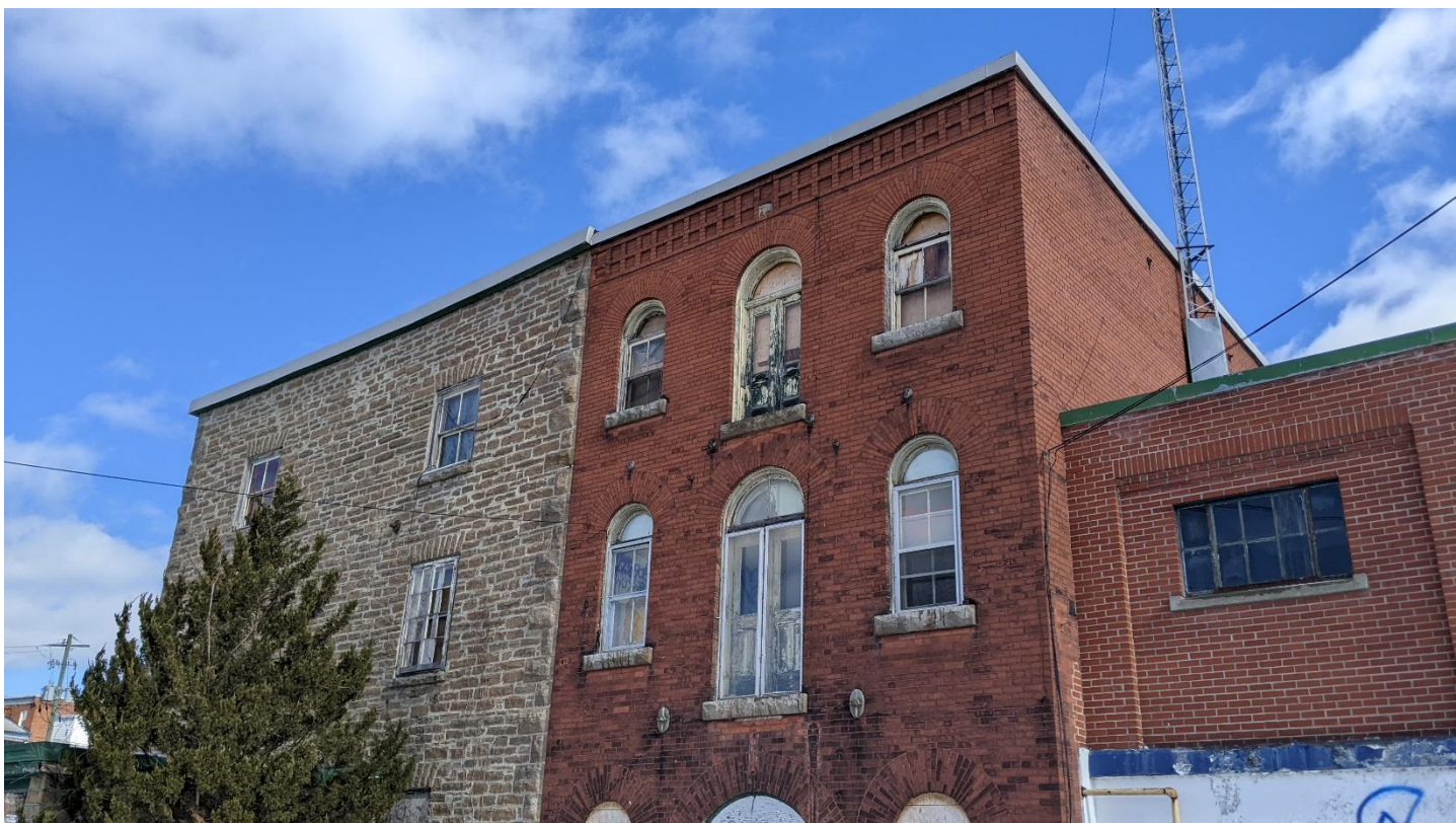
3 Buildings 1, 2 and 3, west façade. Building 2's character-defining elements are especially notable, including the arched windows, stone sills, wooden double-hung windows and decorative cornice. Image: MTBA.
